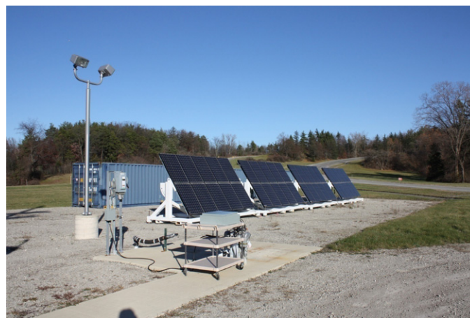
Fig. 1. Picture showing the solar PV battery charging system at the GM Milford Proving Ground. The four arrays have a tilt angle equal to the site latitude plus 15° (57° with respect to the earth's surface). The DC–DC converter box is on the cart in the foreground.
